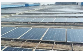
Existing Top Roof Solar
