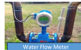
Water Flow Meter
