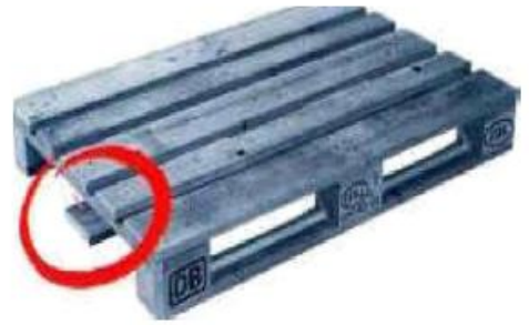
A block is missing or is split so much, that more than one nail or screw is visible.
